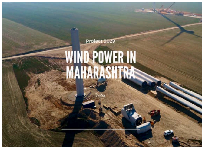
Project 3029: Wind Power in Maharashtra
